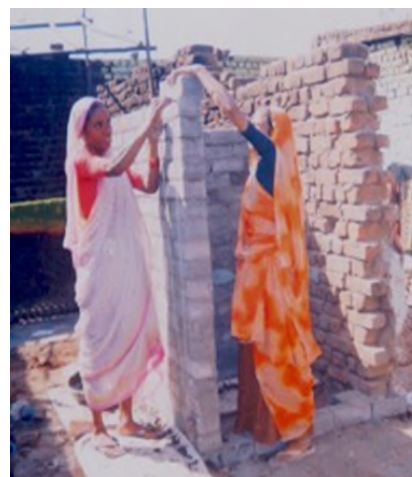
Figure 26: Two women trained in Karmika construct an individual toilet block (cycle 2). Credit: Mahila Housing SEWA Trust
